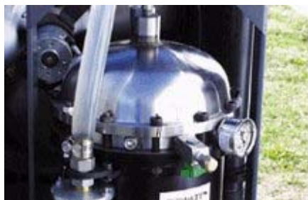
A meter in the foreground shows the temperature, 100°C, of the combustion chamber of Sunpower's Biowatt pelleted biomass generator.
