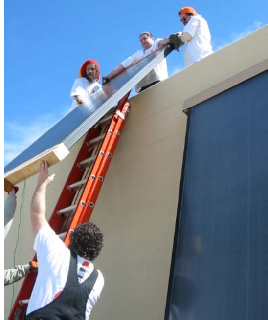
Employees of Cedar Mountain Solar hoist hot-water collectors to the roof of Sonrisa Apartments. The system will save the Saint Elizabeth Shelter $550 per year on heating bills.
