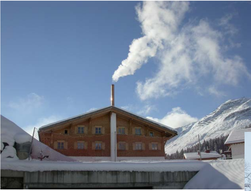
Oberlech, Austria 800 kilowatt Biomass Altitude: 5,500 feet
